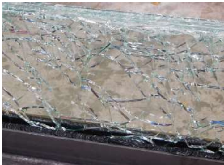
Fig. 13: Part of specimen 2 after having 3 plies damaged. Note the overlapping cracks in successive plies
