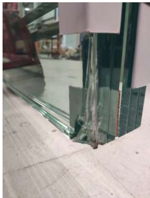
Fig. 4: Transport damage to corner of fin before testing
