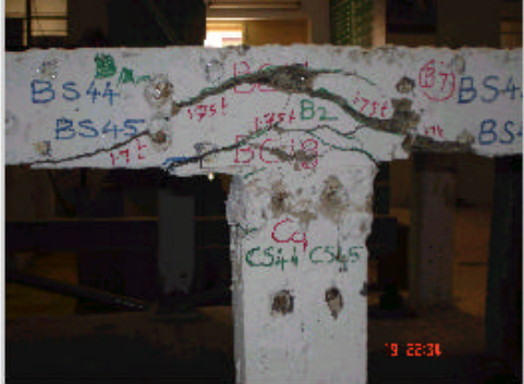
Fig 11: Typical Beams-Column Joint crack in the single long bay
